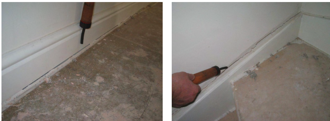
Figure 38 – Shrinkage and cracking of secondary sealing following coheating test
