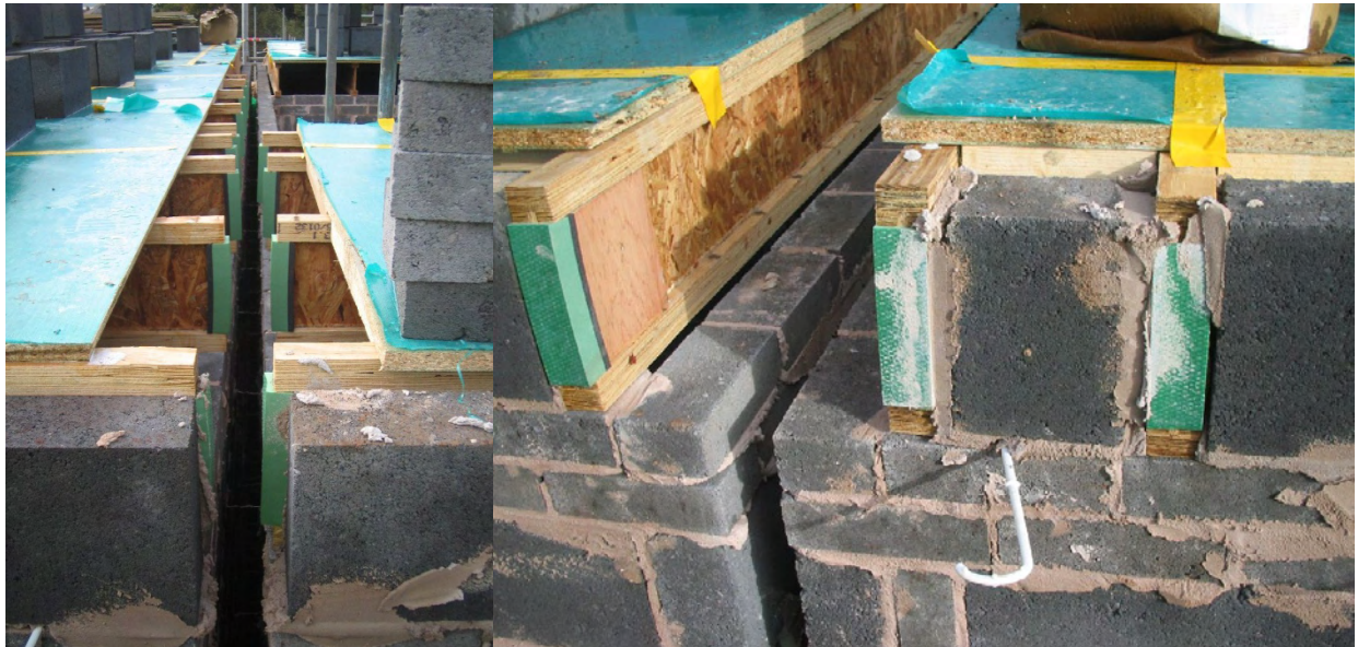
Figure 28 – Mismatch between joist height and block height for built-in joists
