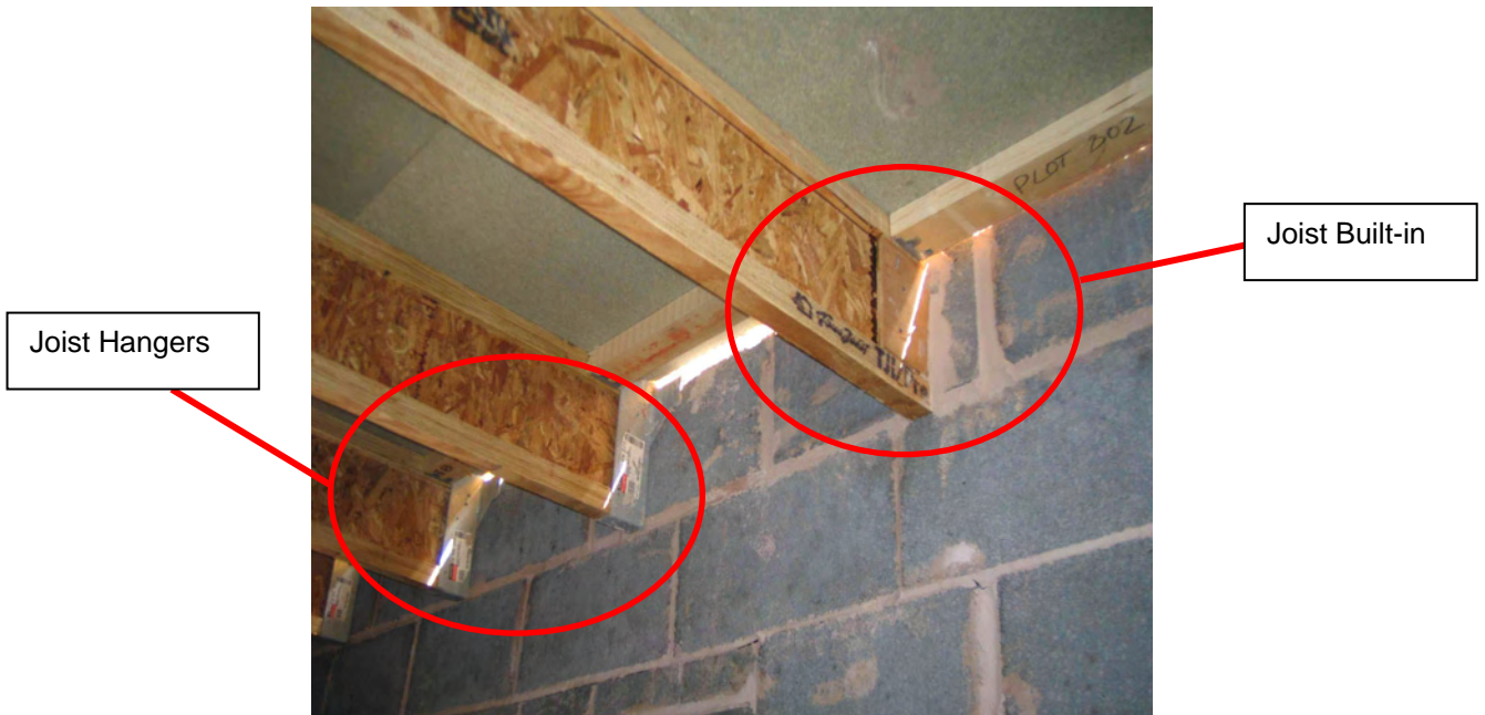
Figure 29 – Intermediate floor built with combination of built-in joists and joists on hangers
