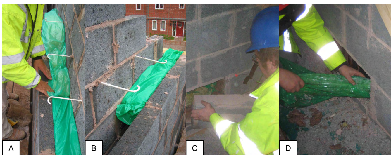
Figure 39 – Horizontal cavity sock being inserted into party wall cavity during construction (A,B) and then being removed again halfway through the coheating test (C,D)
