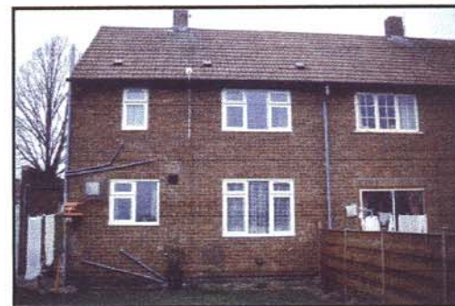
Chapelfield B from back. Note flue for wall mounted heater below living room window, and flue for multi-point water heater to left of kitchen window. Solarimeter is mounted at eaves.
