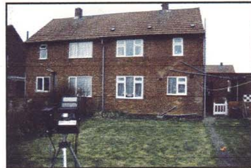
Chapelfield A from back. Note boiler flue to left of kitchen window, and infra-red camera in foreground.
