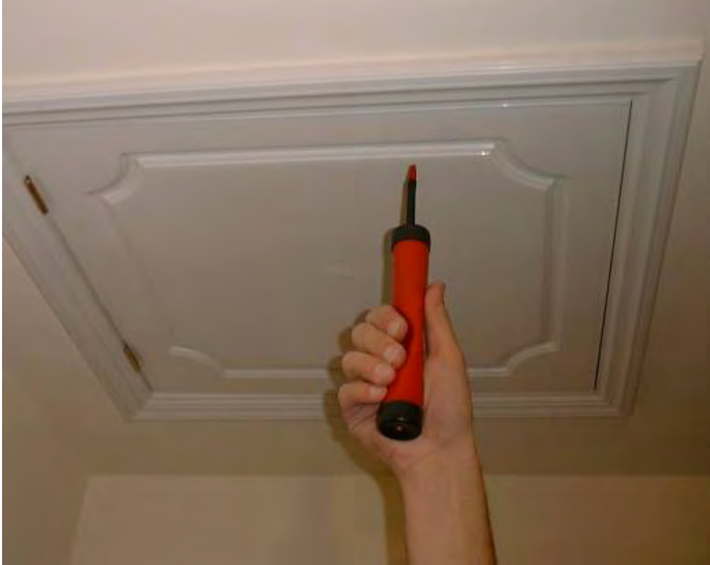
Figure B3 Leakage around the loft hatch.
