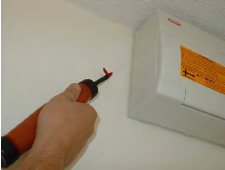
Figure 11 Leaks around electrical fuse box.
