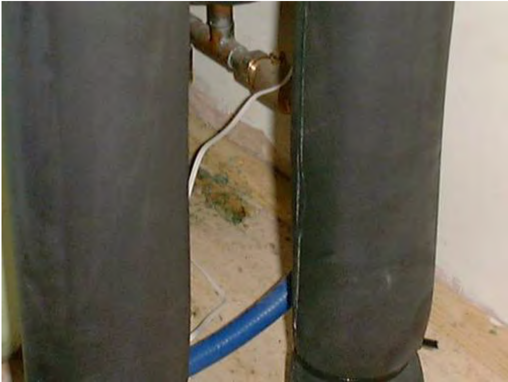
Figure B7 Leakage through service penetrations in the airing cupboard of Plot A.
