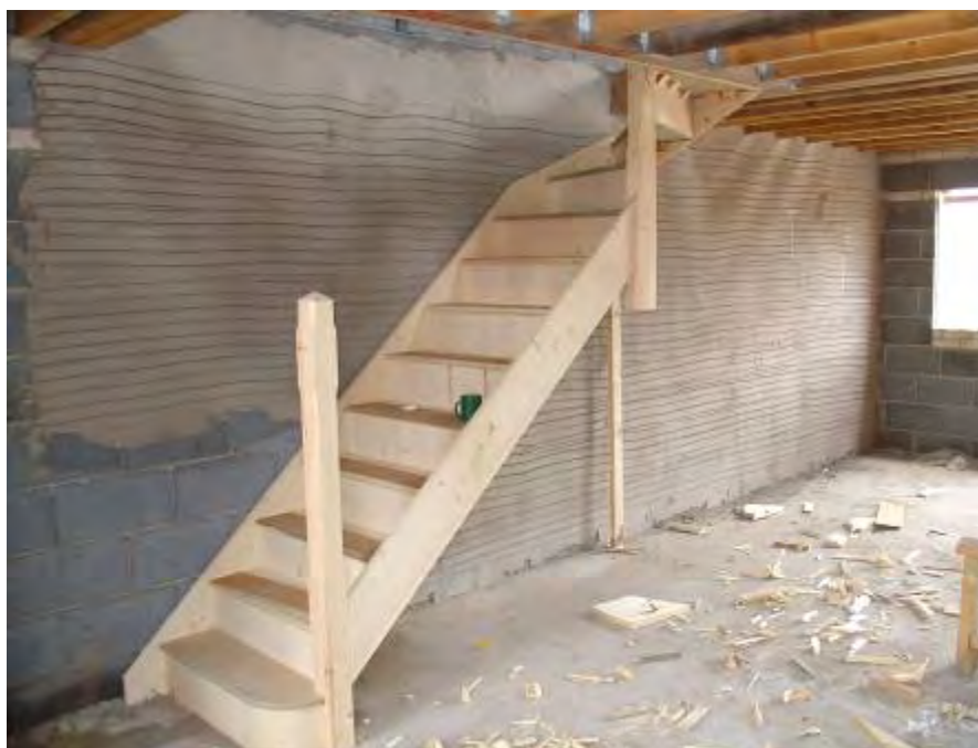
Figure 7 Incomplete scratch coat applied to party walls around stairs.
