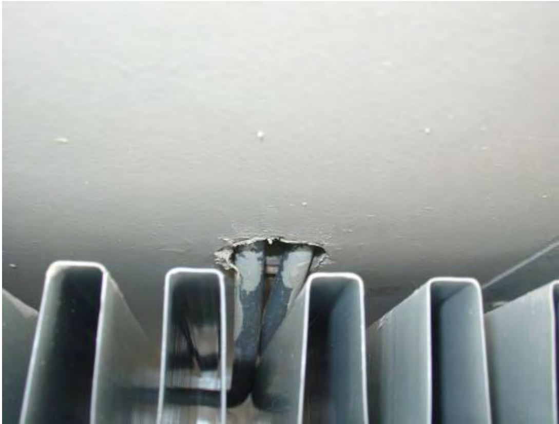
Figure 15 Unsealed pipework penetrations behind radiator.
