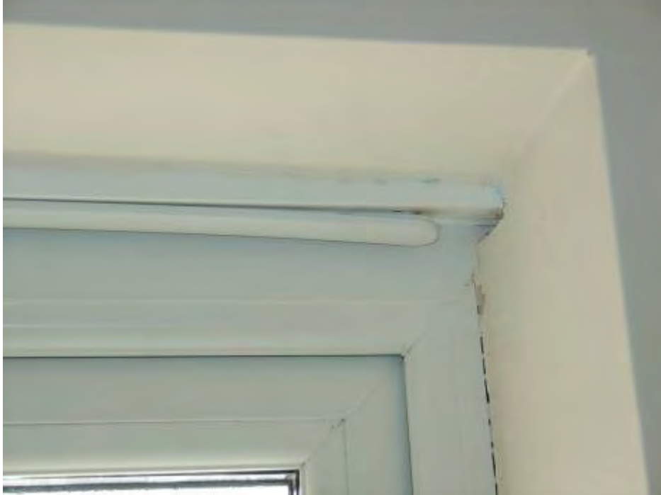
Figure 13 Leaks around poorly fitting trickle vents.
