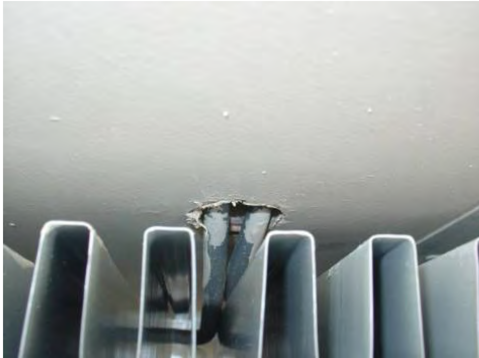
Figure 17 Leaks as pipework penetrates dry-lining behind radiators.
