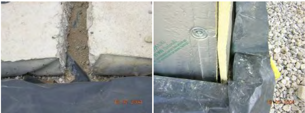
Figure 17 Developer D, Phase 1, the use of removable polystyrene formers created an inconsistent and uneven slab edge, with potential for air leakage at the junction of slab, steel frame and insulation.
