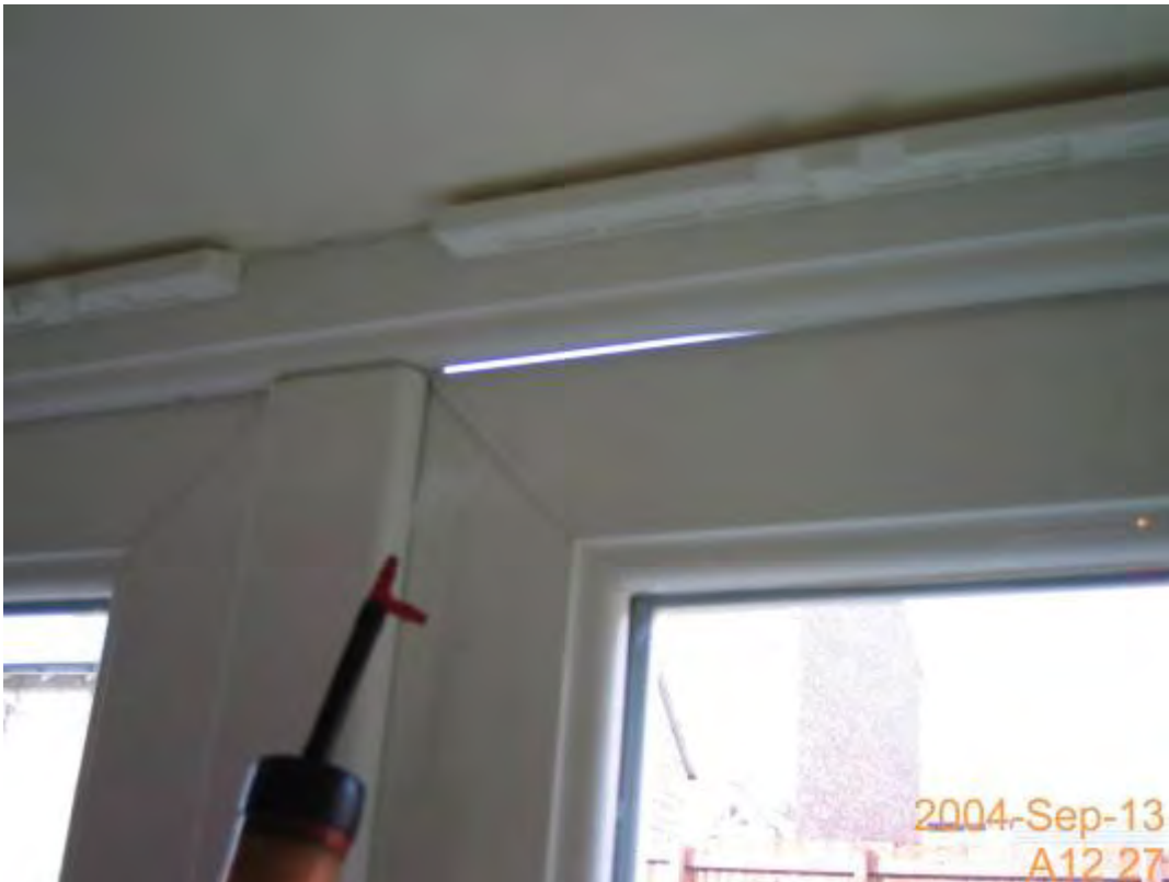
Figure 26 Poorly fitting patio door with visible gap.
