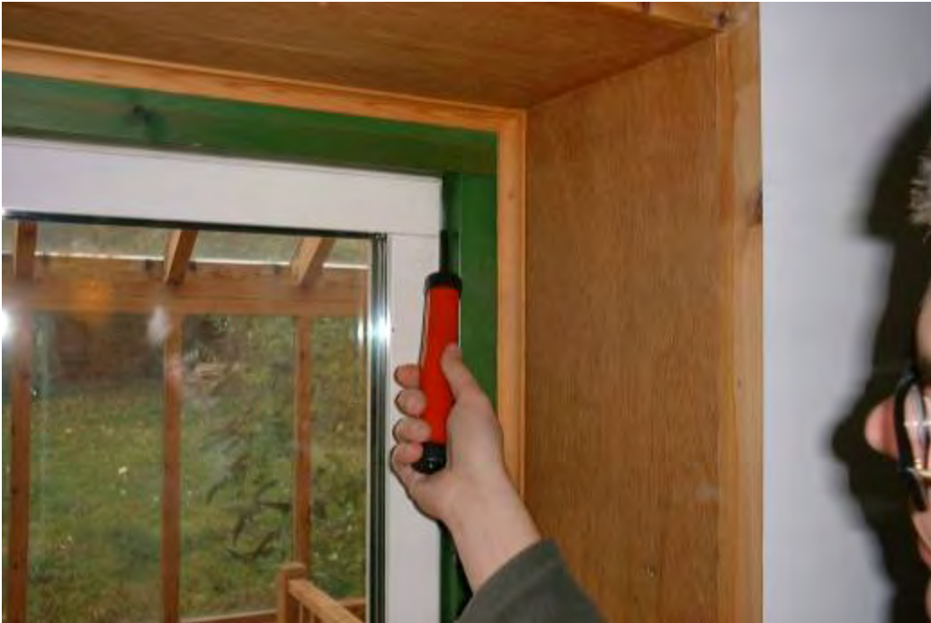
Figure B1 Leakage through opening casement of window.
