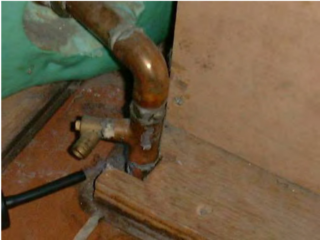
Figure B4 Leakage at pipework penetrations through the ground floor.
