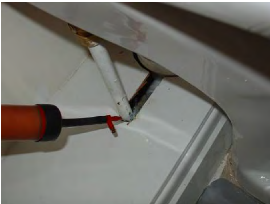
Figure 10 Leaks around water and waste pipes to toilet.
