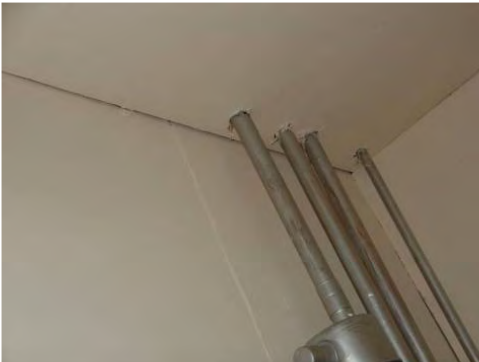
Figure 24 Leaks around service penetrations and at ceiling junction in boiler cupboard.
