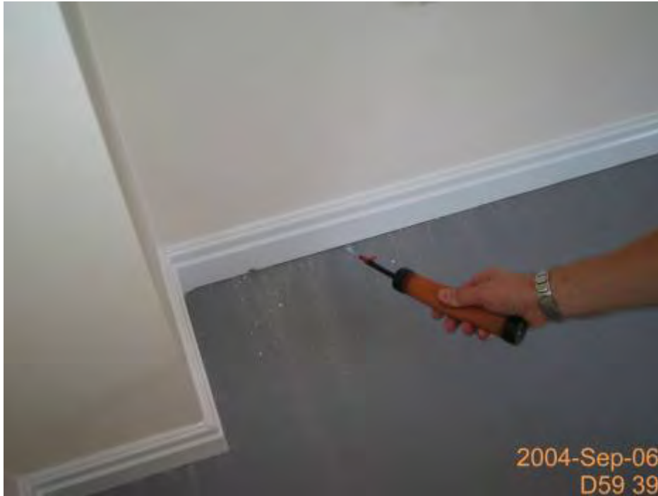
Figure 29 Leak at gap between skirting board and ground floor.
