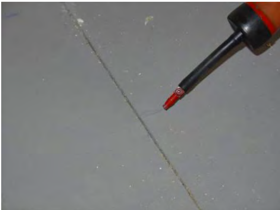
Figure 20 Leaks at the junction between flooring panels.
