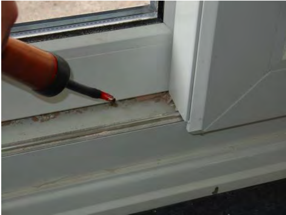
Figure 15 Leaks around bottom of patio doors.
