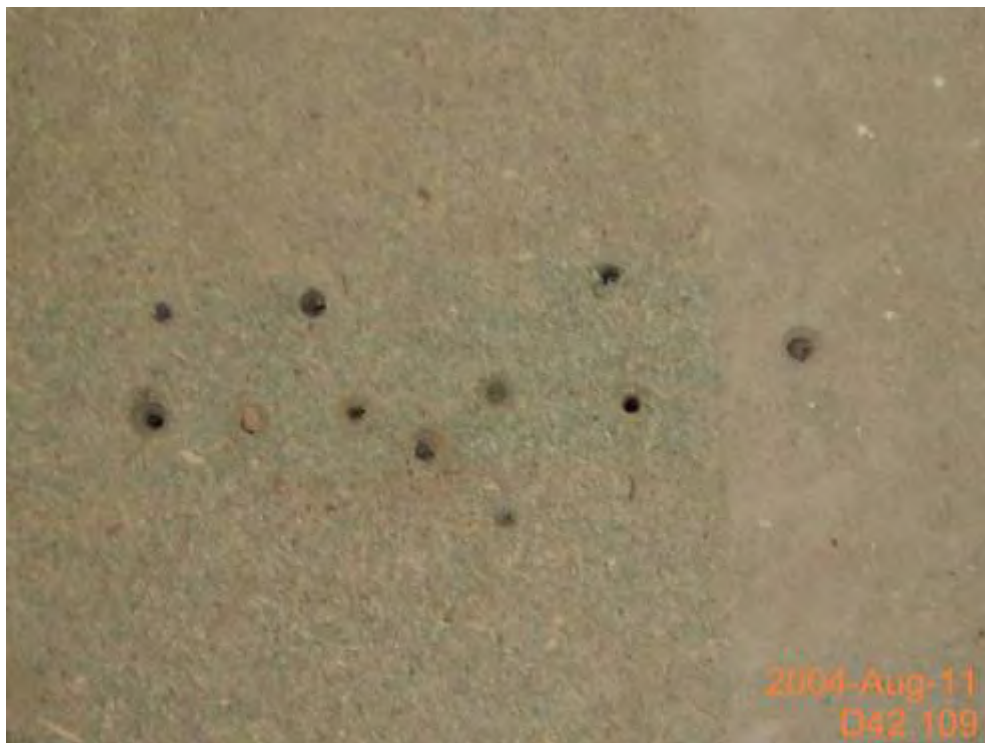
Figure 21 Screw holes in the flooring panels.
