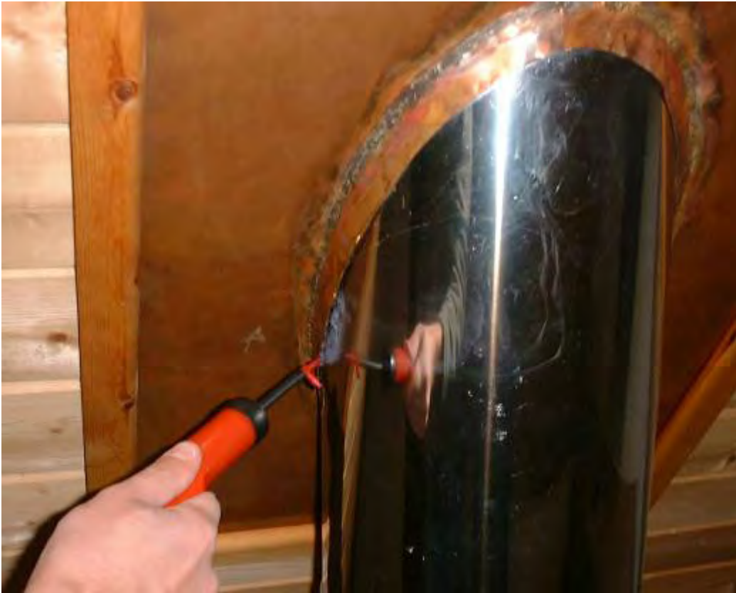
Figure B3 Leakage at the junction between the vent stack and the ceiling.
