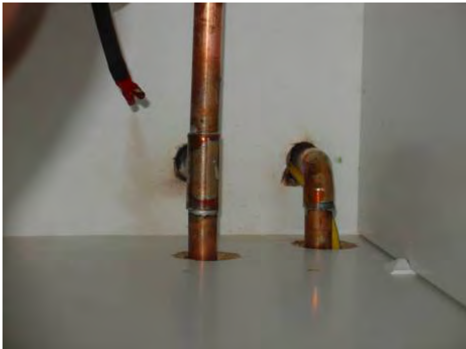
Figure 7 Leaks around water pipes.
