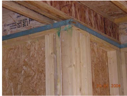
Figure 3.76 High timber concentration at corner post.
