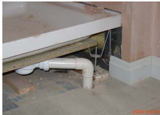
Figure 3.83 Plasterboard finish cut away to enable the shower tray to be inset, giving access to the structural space.
