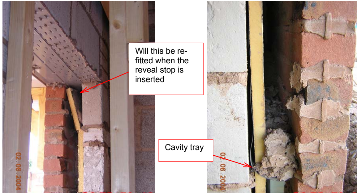
Figure 3.44 Partial-fill cavity insulation – gaps and mortar build-up on cavity tray.
