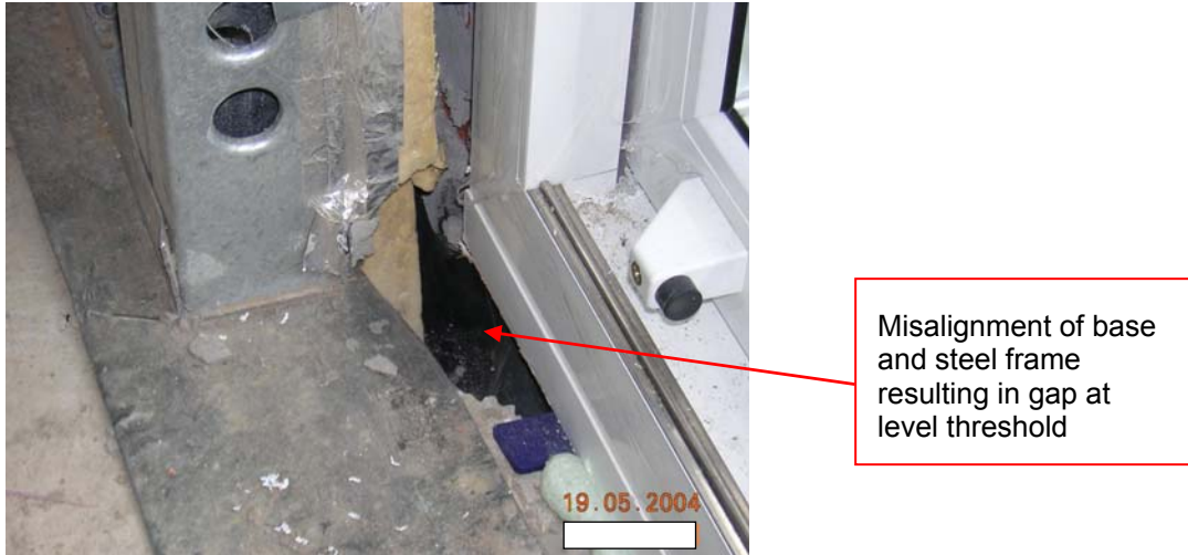
Figure 3.21 Gap at level threshold.
