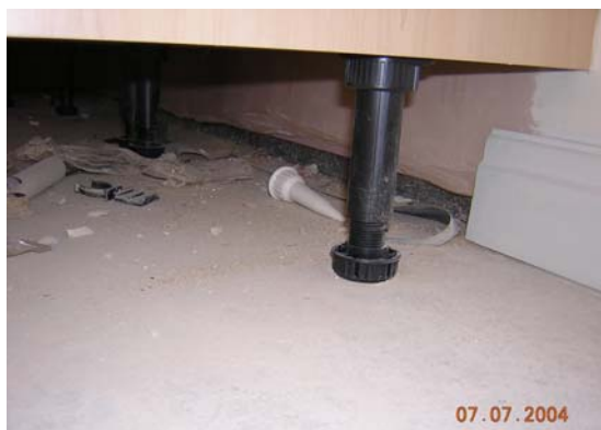
Figure 3.82 Plasterboard finish stopped short of the floor under kitchen fittings.
