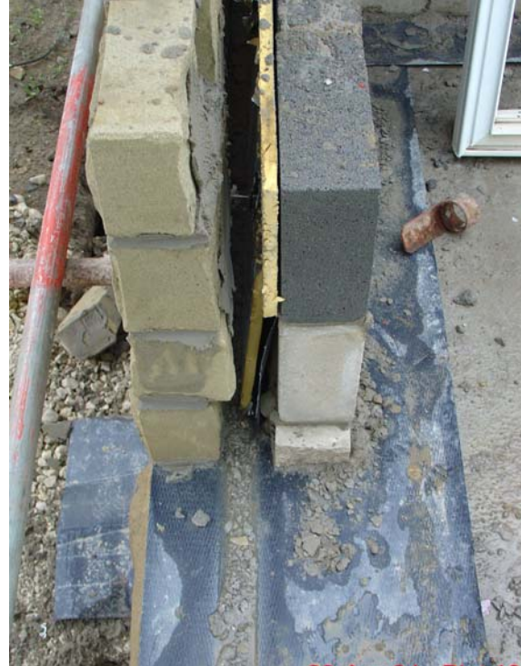
Figure 3.69 Partial fill insulation displaced by cavity tray resulting in gaps around insulation.
