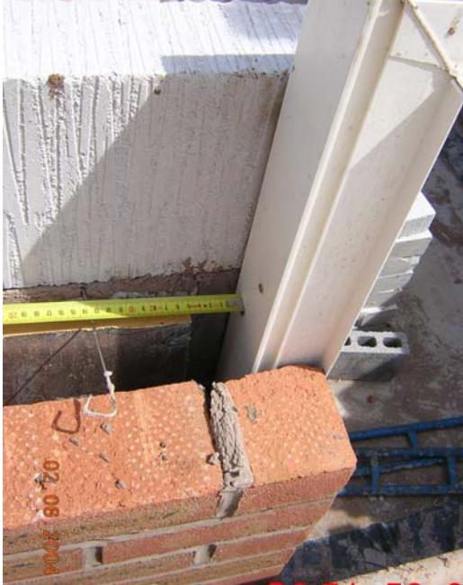
Figure 3.42 Gap observed between cavity closer and partial-fill cavity wall insulation.
