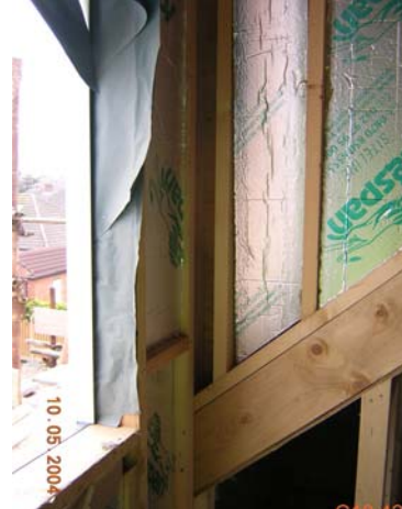
Figure 3.66 Omission of insulation at small strip in the corner.
