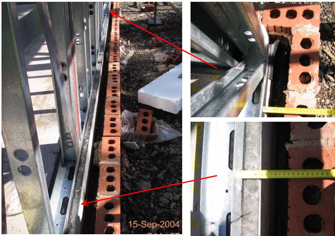
Figure 3.18 Slab not square in steel frame construction.
