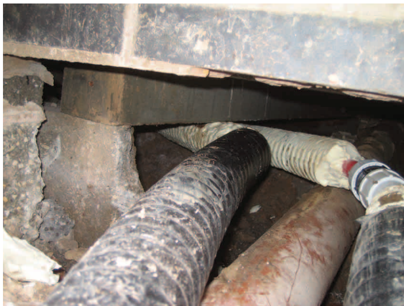
Pipe work below the floor showing outer protective sheath and insulation stripped away to enable the pipe to be bent
