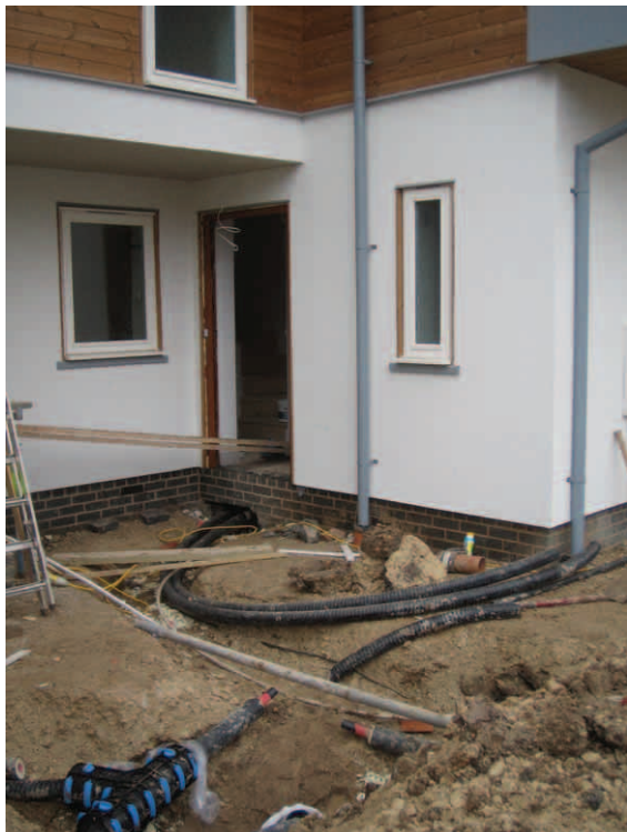
District heating pipe being fed under ground floor of dwelling through hole in foundation wall
