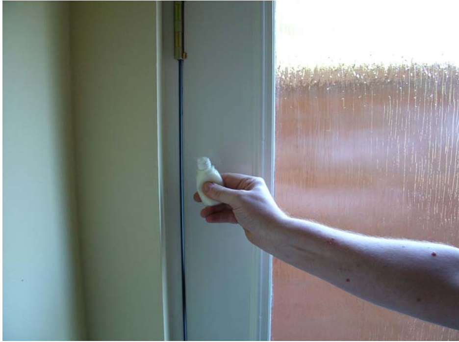
Figure 4 Air leakage through gaps around poorly fitting back door.
