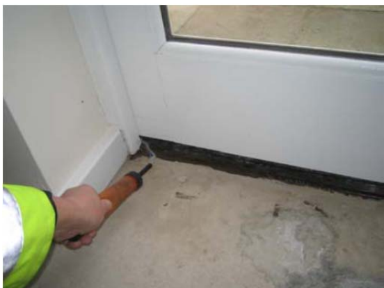
Figure 4: Air leakage under patio doors.
