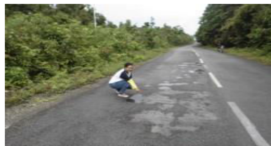
Figure 3.2a. Damage type Hole with high damage level on Biak-Korem-Supiori road
