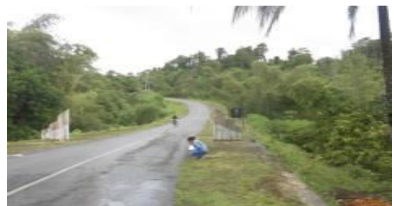
Figure 3.2b. Type of crack fracture edge with moderate damage level on Biak-Korem-Supiori road
