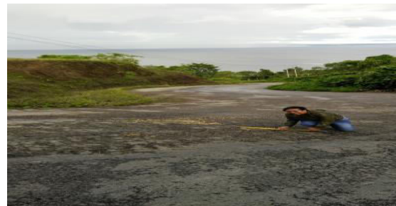
Figure 3.1c. Type weathering damage and raveling With high damage levels on the Aminweri-Yendoker road
