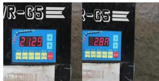
Figure 7. Flow Control Equipment and Frequency
