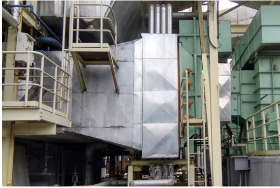
Figure 1. Steam coil air heater.
