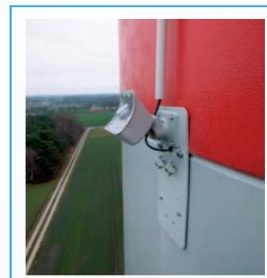
Latest DTBirdV8 model installation on a concrete WTG. 2 to 8 HD cameras can be installed per tower.
