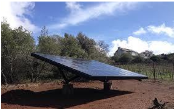
Figure 2. Solar installation isolated to public grid.
