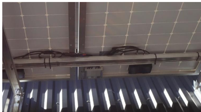
Figure 19: PV system with DC-DC optimizer [19]
