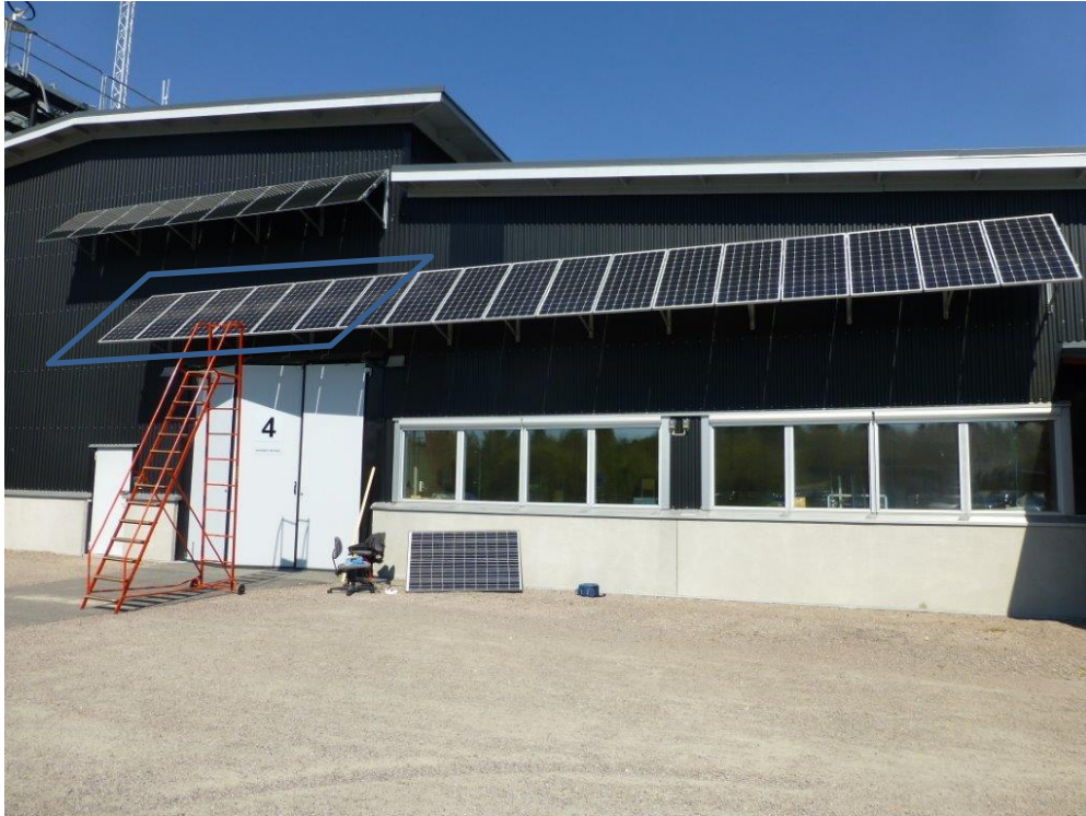
Figure 26: String of six modules with bypass diodes at HIG laboratory
