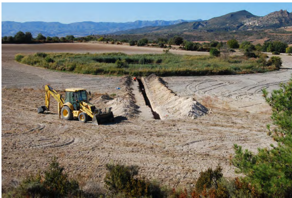
Fig. 3. View towards the north-west of trench T4 excavated with a radial orientation from the edge of the Basturs Small Lake. A reference orthogonal grid with a spacing of 1 m on the right wall of the trench (northern wall) was used for accurate logging of sedimentological and deformation structures. The excavator is ca 6 m from the front to the back bucket.
