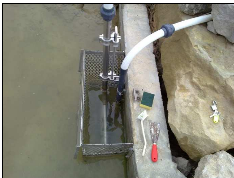
Fig. 3-3. Details of EC-meter and Nitratax equipments installed in the gully.
