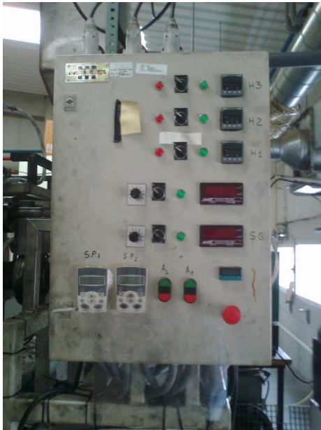
Figura A.11 Panel de control
