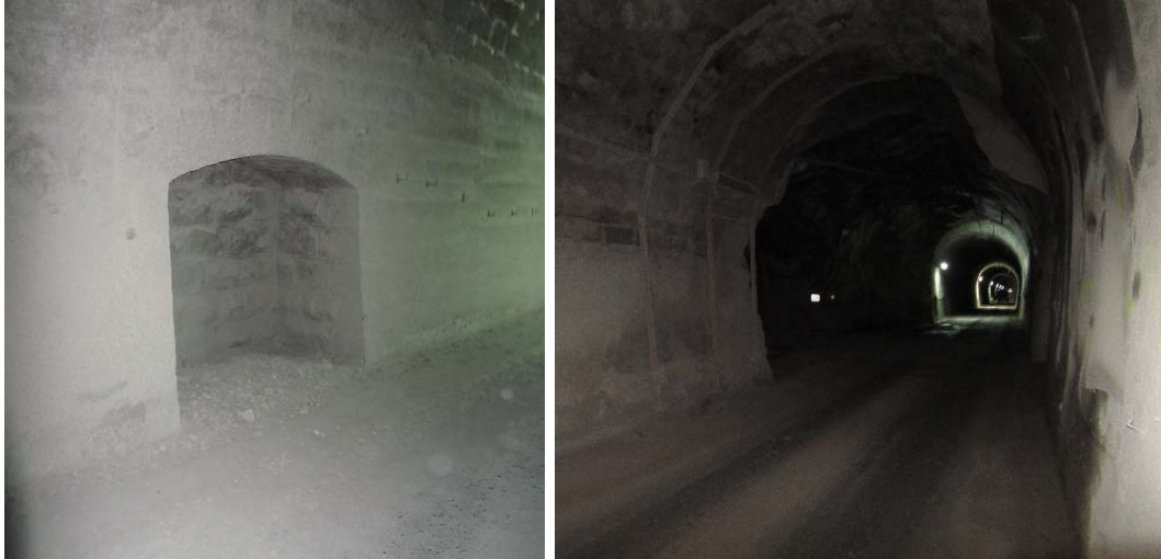
(a) (b) Figure 2. Small Vaults in the tunnel (a), and galleries (b).
