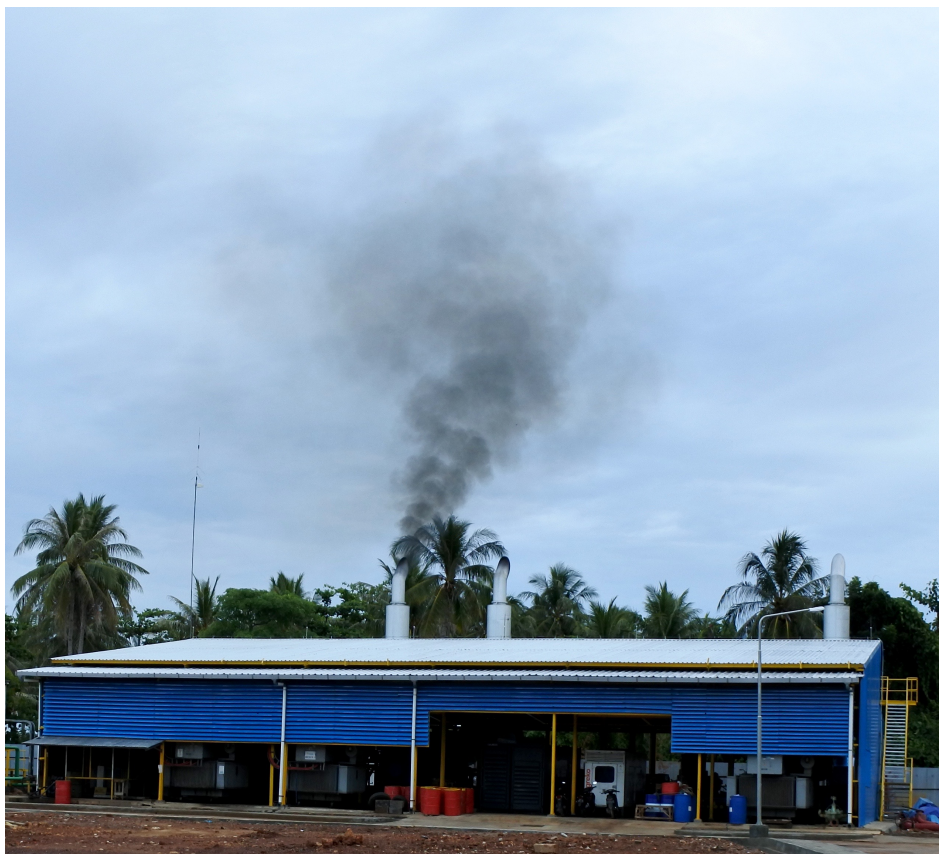
Figure 18: The diesel power plant on Karimunjawa main island
