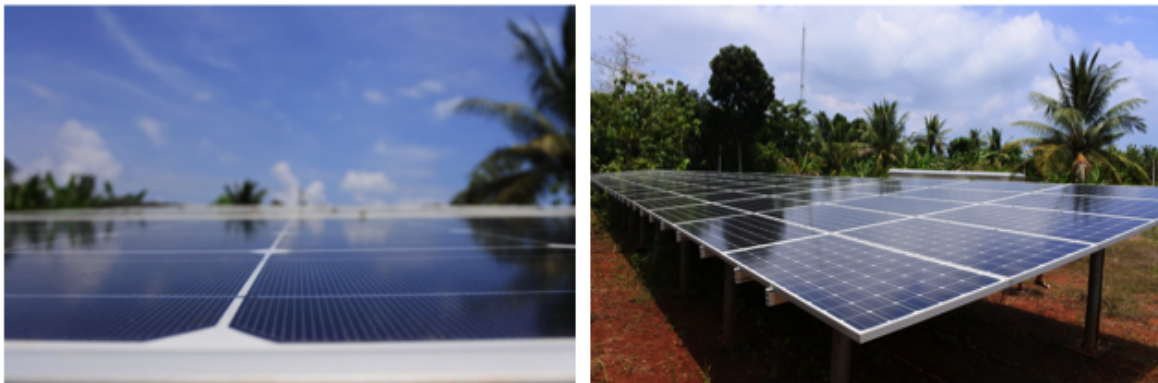
Figure 20: Solar panels on Parang island
