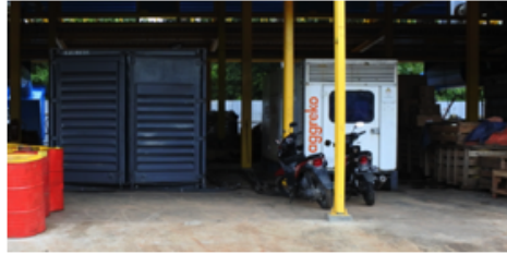
Rental diesel engines, to the left 1x 500kW and to the right 1x 305kW
