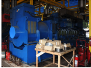
2x 2.2 MW diesel engines
