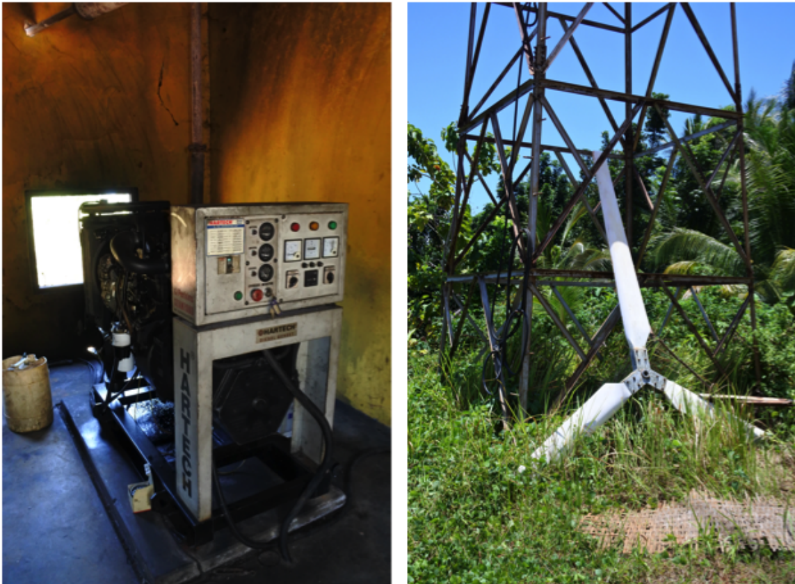
Figure 25: Diesel engine and broken WTG
