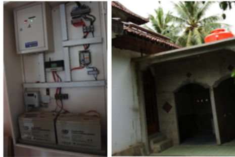
To the left, 2x Solar Home systems and to the right 8x solar powered fresh water pumping systems
