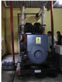
6x 500kW diesel engines
