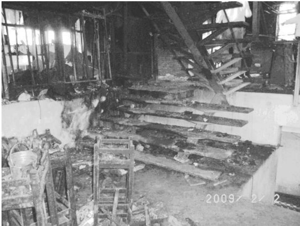
Image 6: The staircase leading to the entrance hall of the Santika nightclub; Image taken from [65]
