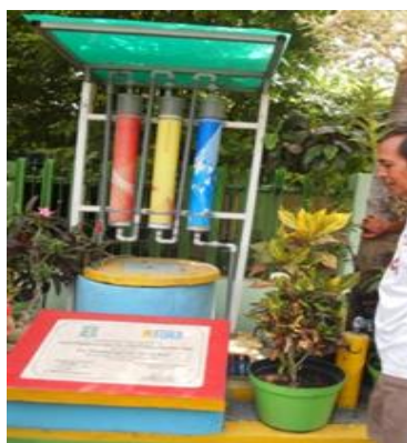
Figure 3. Wastewater Treatment Plant (IPAL) Source: field survey
