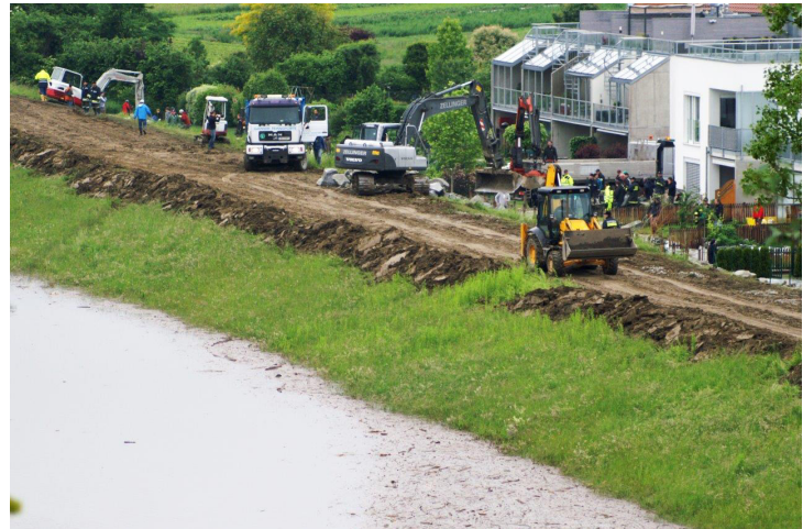
Figure 4. Flood dam in Ottensheim needed heavy adjustments during the flood 2013 as it almost broke after it started to leak at several spots along the dam (Foto: Hagenauer)
