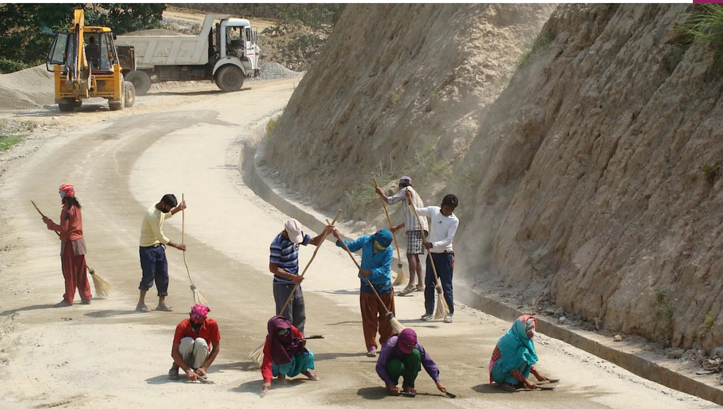
Migrant workers from Kapilbastu and Banke doing preparatory work for blacktopping the road from Kathmandu to Nuwakot District
