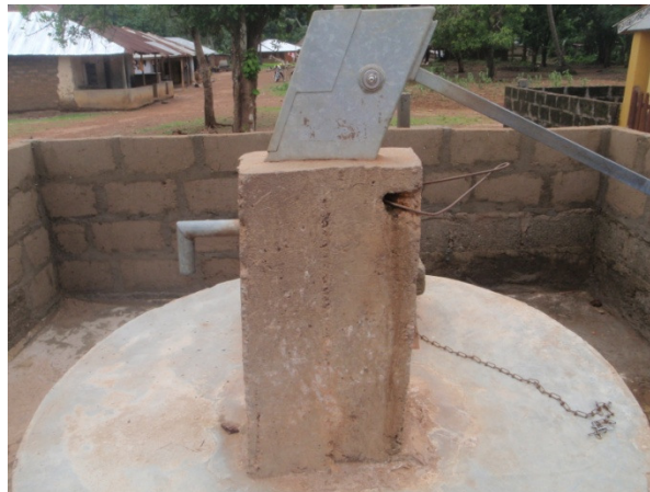
Figure 610 Concrete Security Casing in Rowala Village
