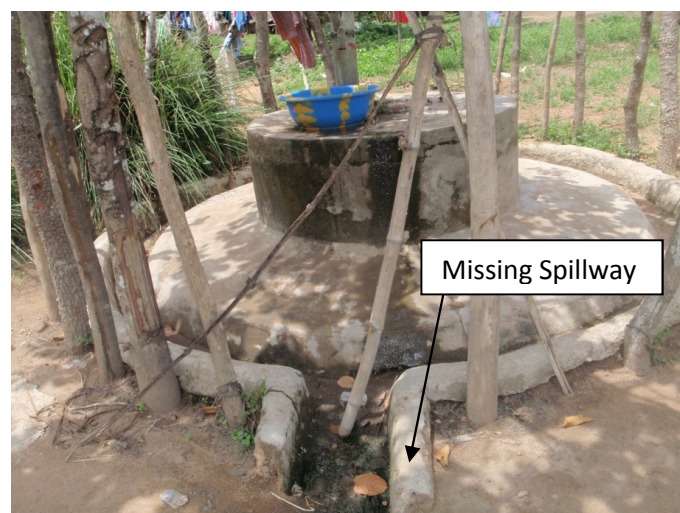
Figure 59 Two House village well - missing spillway
