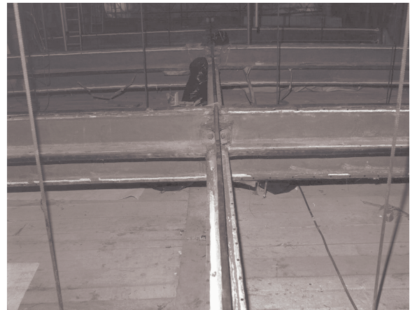
Shadwell station struts, London Underground
