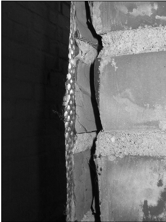
Figure 13 – De-bonding of clay wall
