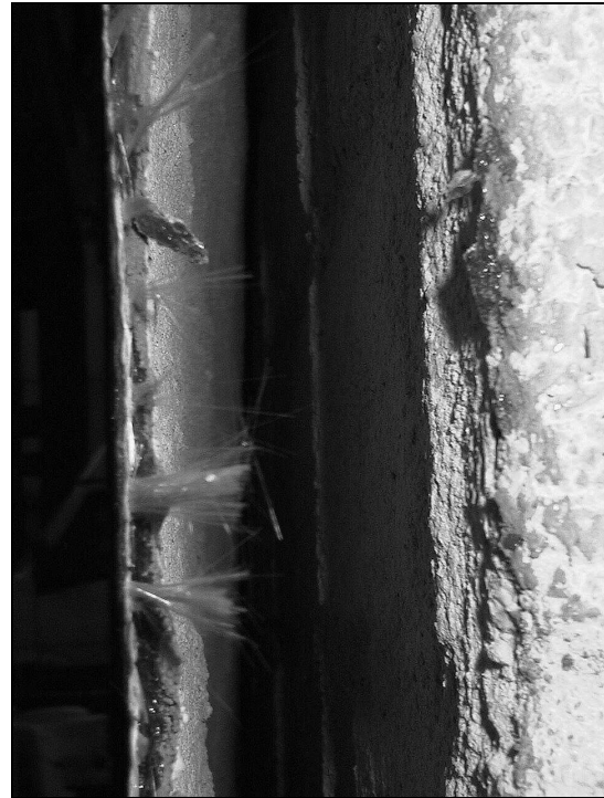
Figure 14 – De-bonding of concrete wall
