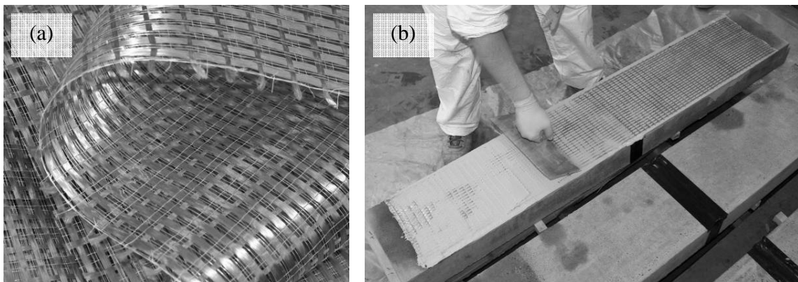
Figure 2. (a) Open-weave PBO fibre fabric and (b) installation of the first layer of the FRCM system on one of the beams
