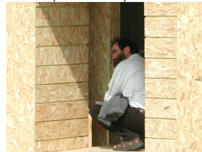
Figure 10: This man stays inside the passage between the sides of the wall during all the phone conversation, the head is orientated perpendicularly to the sides
