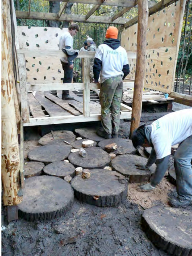
Fig. 10 - Student Live Project constructing an outdoor classroom from locally sourced timber [Photo: Prue Chiles]
