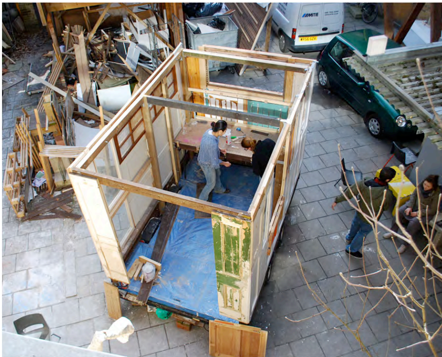
Fig. 22 - Student construction project for a mobile home, Studio 3 ASD [Photo: Sandra Denicke Polcher]
