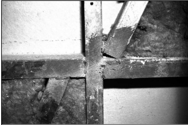
Figure 8. Wall panel removed, showing no trace of corrosion on the members after 15 years (the connections are coated in zinc-rich paint)
