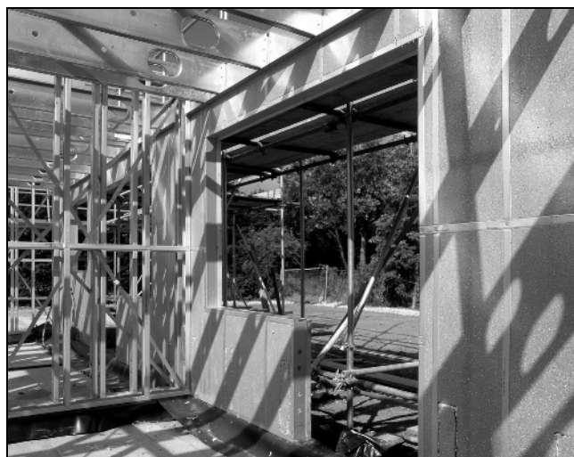
Figure 1. Light steel framing in housing development, using bonded expanded polystyrene between the C sections (Fusion Building Systems)
