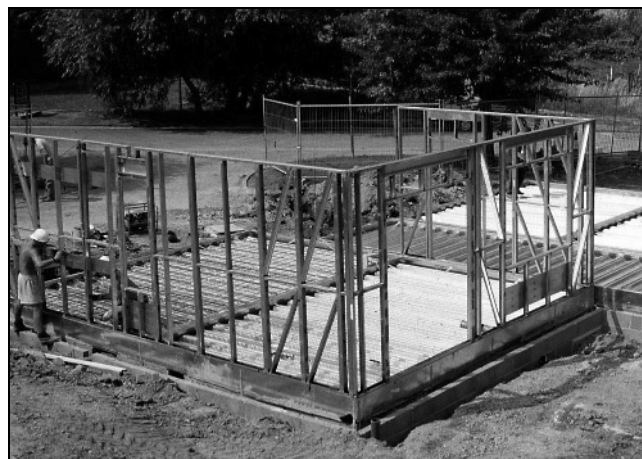
Figure 15. Ground-floor system in the OBU house (using composite decking and perimeter C sections)
