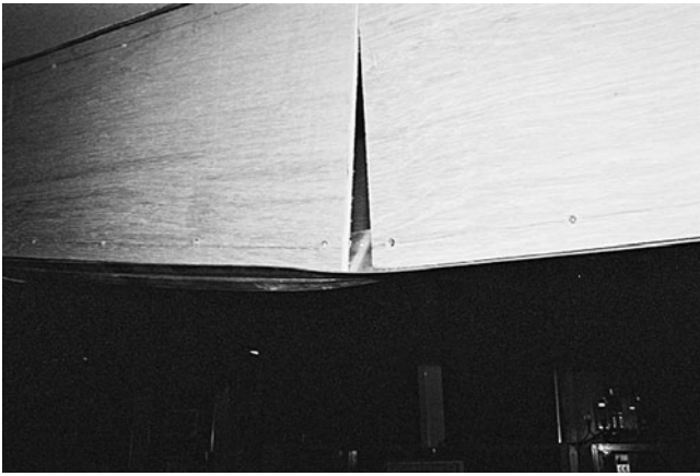
Figure 5. Local deformation at joint in plywood web
