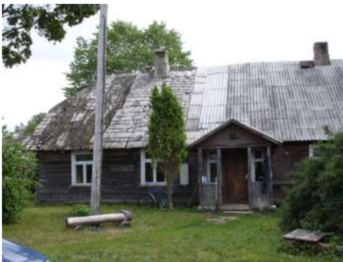
Figure 1b An old rural house in a poor state of repair
