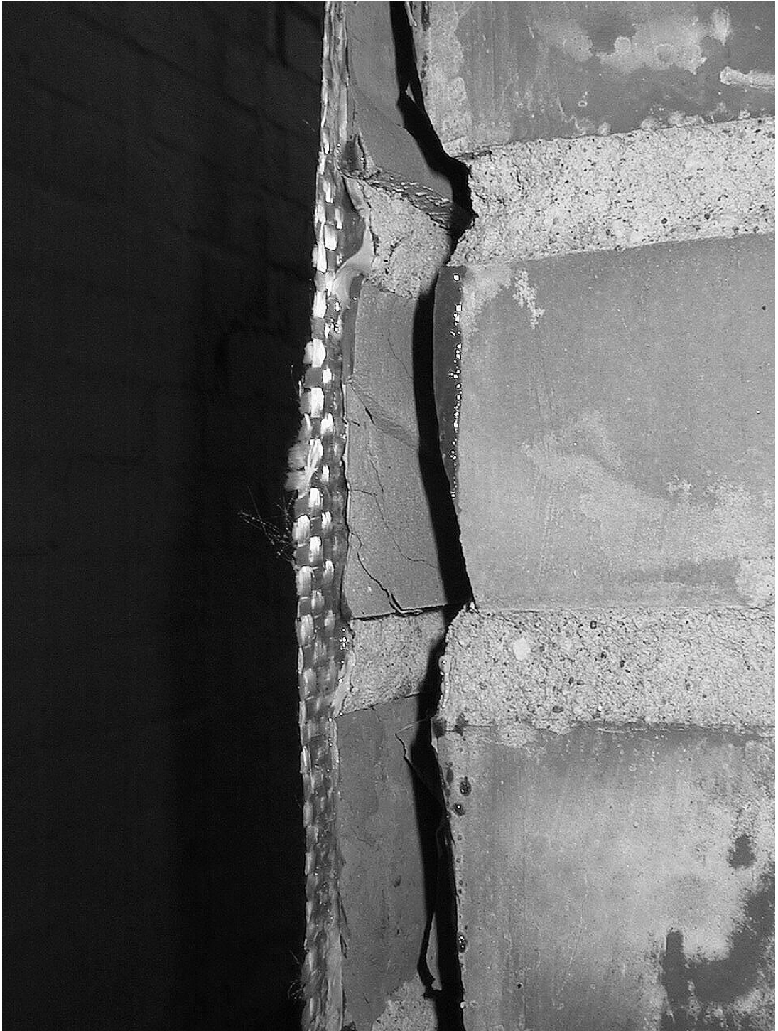
Figure 11 - Failure of the GFRP-masonry interface in a clay panel.
