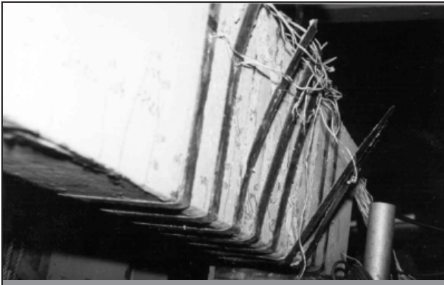
Figure 13. FRP-plated RC beams: debonding of FRP U-jackets
