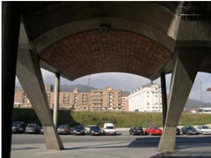
Figure 4. The reinforced concrete buttresses supporting the roof, fitted with a pin connection at their lower end.
