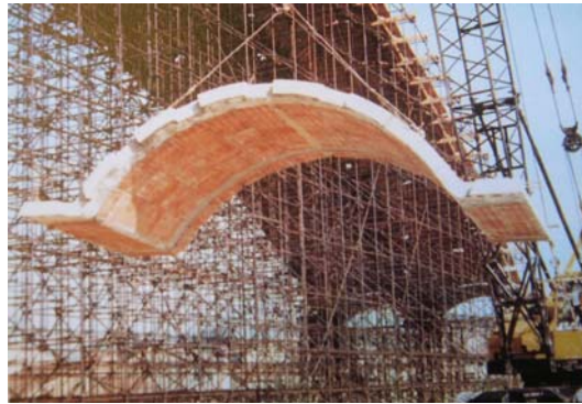
Figure 5. Centering and assembly of the roof of the Oviedo Sports Hall [Colegio 2004]
