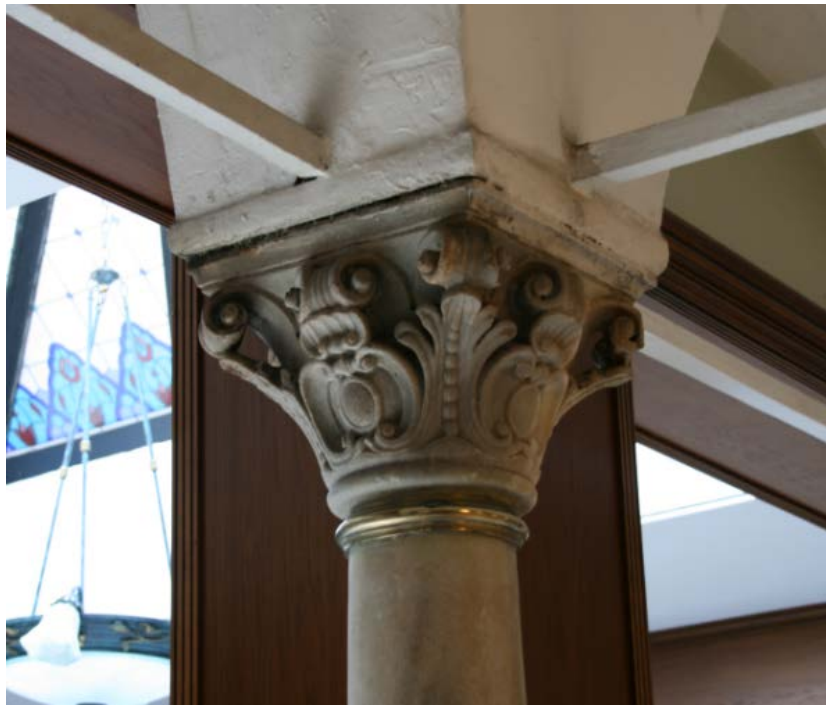
Figure 417. Hamidiye Complex, column of the vestibule connecting the masjid to the madrasa.
