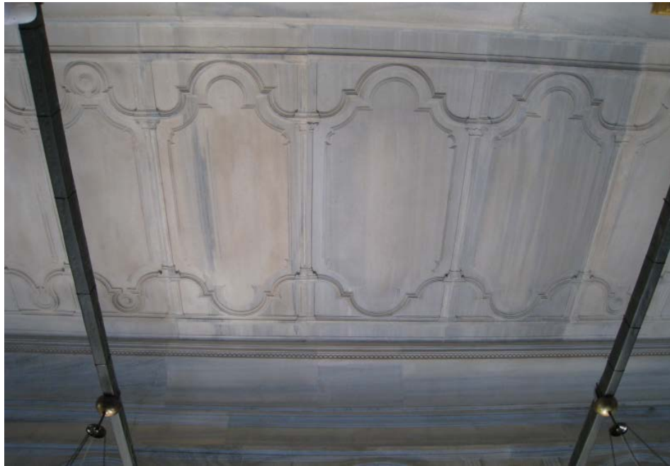
Figure 325. Nuruosmaniye Mosque, Marble ceiling panels on the underside of the southwest gallery.
