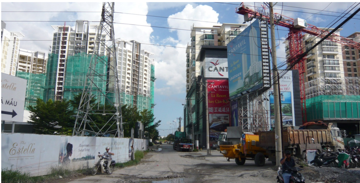
Fig. 8. Apartments developed by a Singaporean joint venture (left) and by a Korean joint venture (right) Source: Photograph by the author
