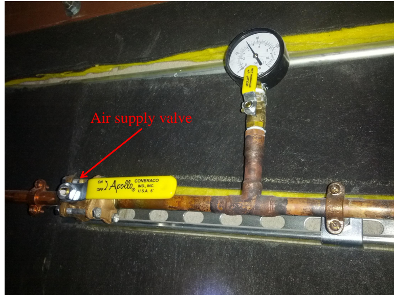
Figure A.8: Photo of a valve responsible for controlling the flow of pressurized gas from the building supply line. One valve controls flow to the room air springs, and another controls flow to the table air springs.
