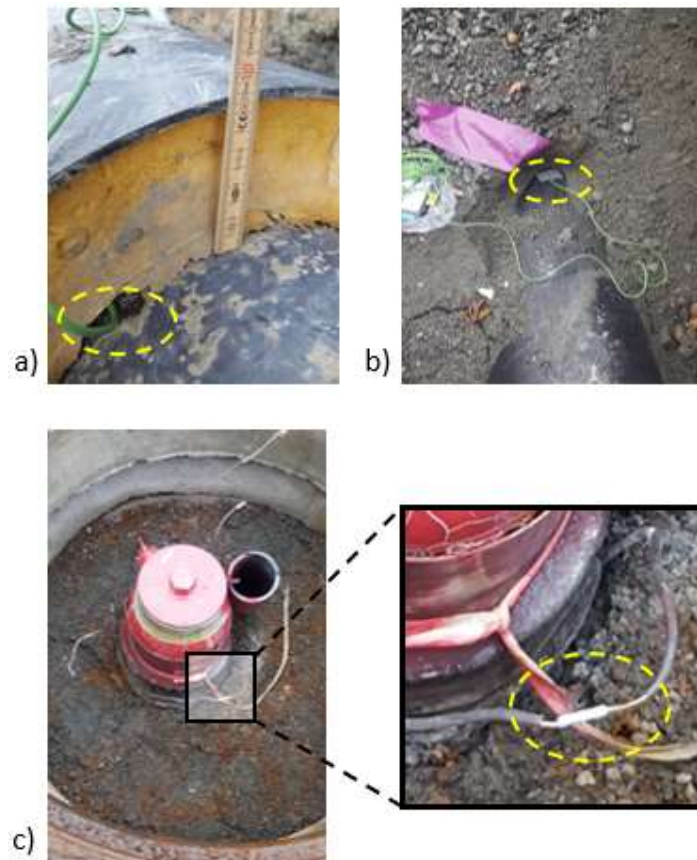
Fig. 9. a) TC for measuring T_s inserted under the PUR. b) TC for measuring T_{cp} attached to the casing before fillings were laid back. c) Coupled copper wires next to a valve in a manhole.
