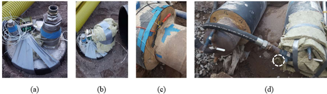
Fig. 13. (a) Valve at point B with TC attached on the valve to the right. (b) The same valve after insulation with mineral wool. (c) The service pipe at the excavation with TCs measuring T_s and crocodile clamps on the ends of the copper wires, connected to a multimeter. (d) The same pipe (supply), to the right in photo, after insulation with mineral wool. White dotted circle shows the valve on the flexible pipe which was switched off for the shutdown.
