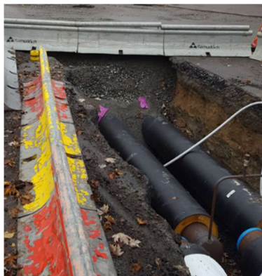
Fig. 8. The excavation with two single pipes, of which the field test was carried out on the supply pipe (to the right). The small uninsulated vertical interconnected pipe can be seen between supply and return pipe in the photo.
