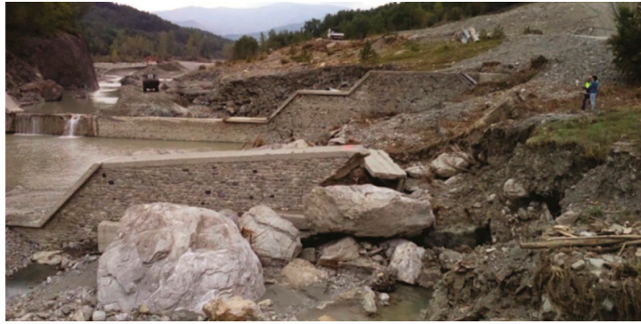
Figure 11. The Sassi Neri check dam after the flood event (from downstream). The flow circumvented and damaged the structure on the left.
