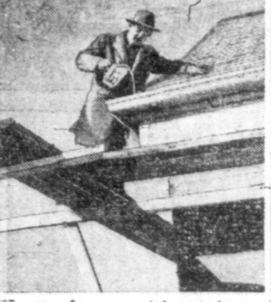
THE alert home builder will keep watch over things as his house goes up. Here are some salient points to be checked. Equally important, before actual building begins, are neighborhood, services such as water, sewers, gas and electricity and nature of the soil.
