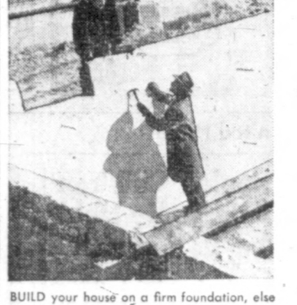
BUILD your house on a firm foundation, else it will sag. Waterproofing prevents dampness from seeping through.
