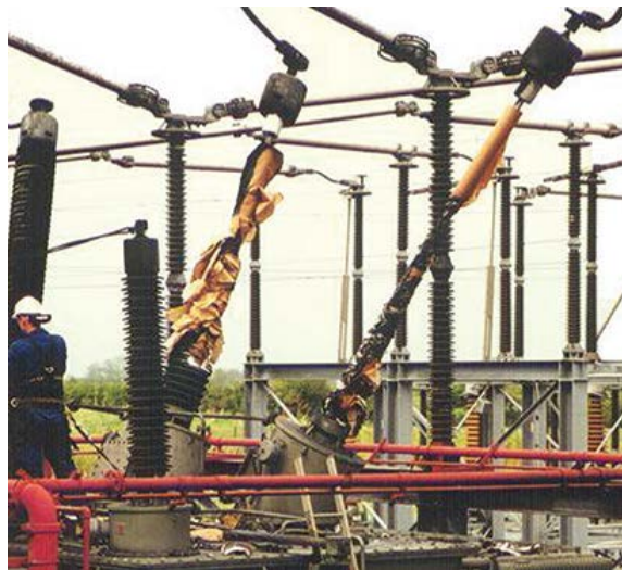
Figure 2-4: Damaged bushings. Reproduced from ref. (18).
