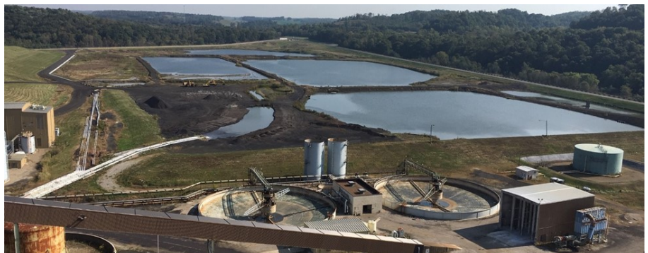
View of the fly ash handling system from the top of the Number 6 unit
