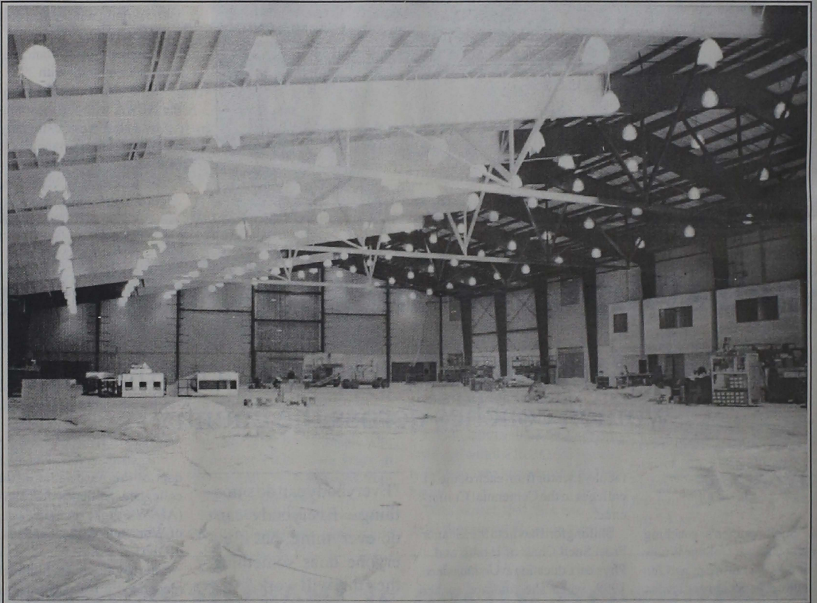
Construction on the Floy-Lewis Bakes Field House continues on the Ursinus campus. The completion of the facility is scheduled for mid-March. Photo by Joe Laskas.
