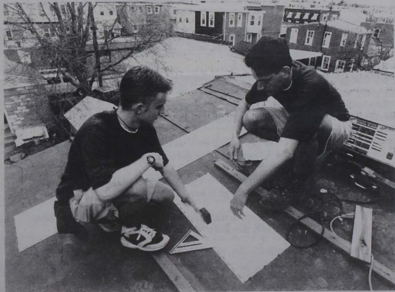
Two Ursinus student volunteers begin to place shingles on a roof of one of the Habitat for Humanity houses in Norristown. The second annual Spring Service Day was held April 20.
