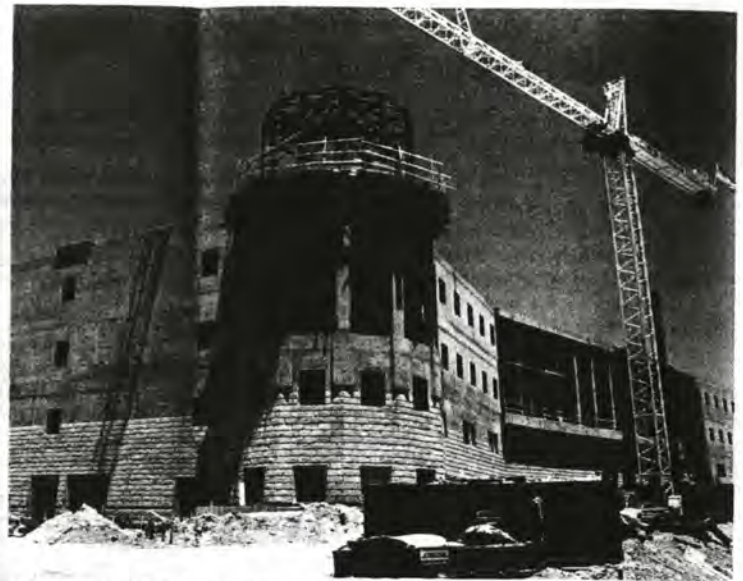
Opening in Fall 2003, the Donald Pearce Shiley Center for Science and Technology will be the largest building on campus.
