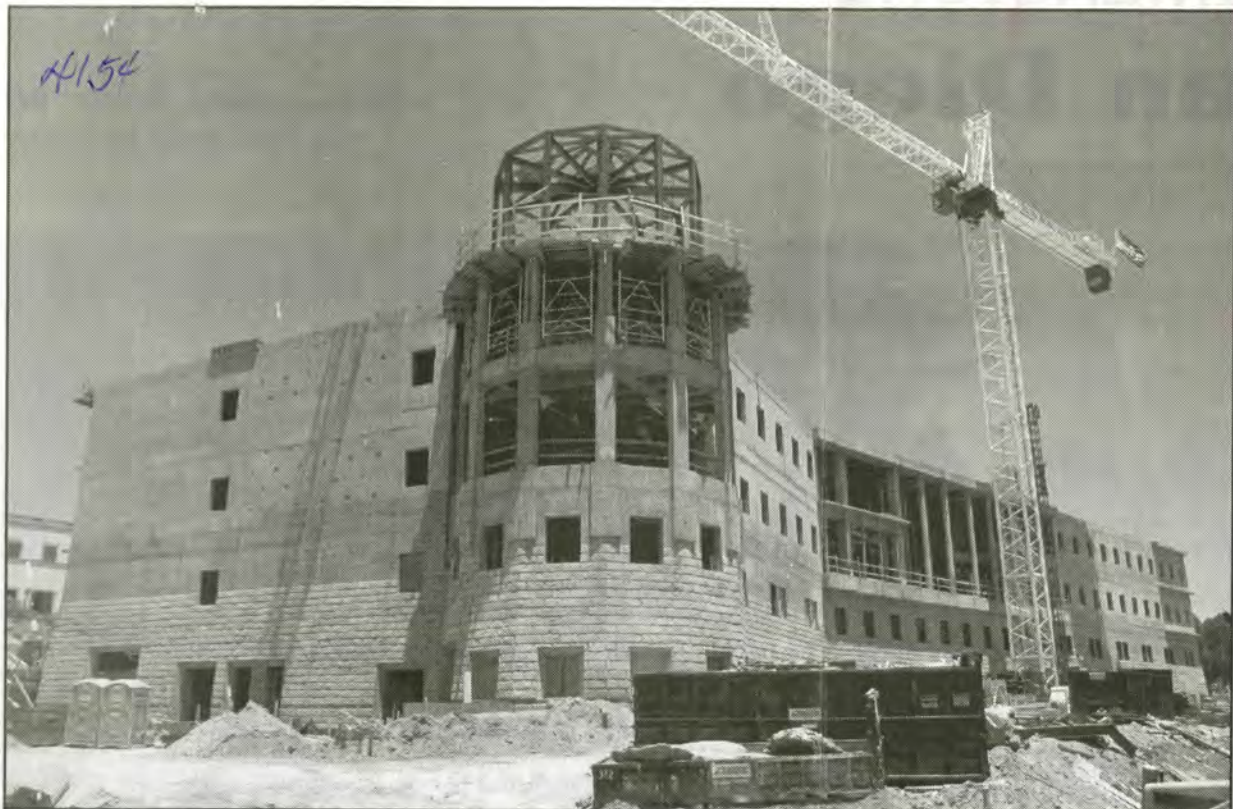
The 150,000-square-foot Donald Pearce Shiley Center for Science and Technology will be the largest academic building on USD's campus, when it opens in the fall 2003. Photo credit: Brock Scott
