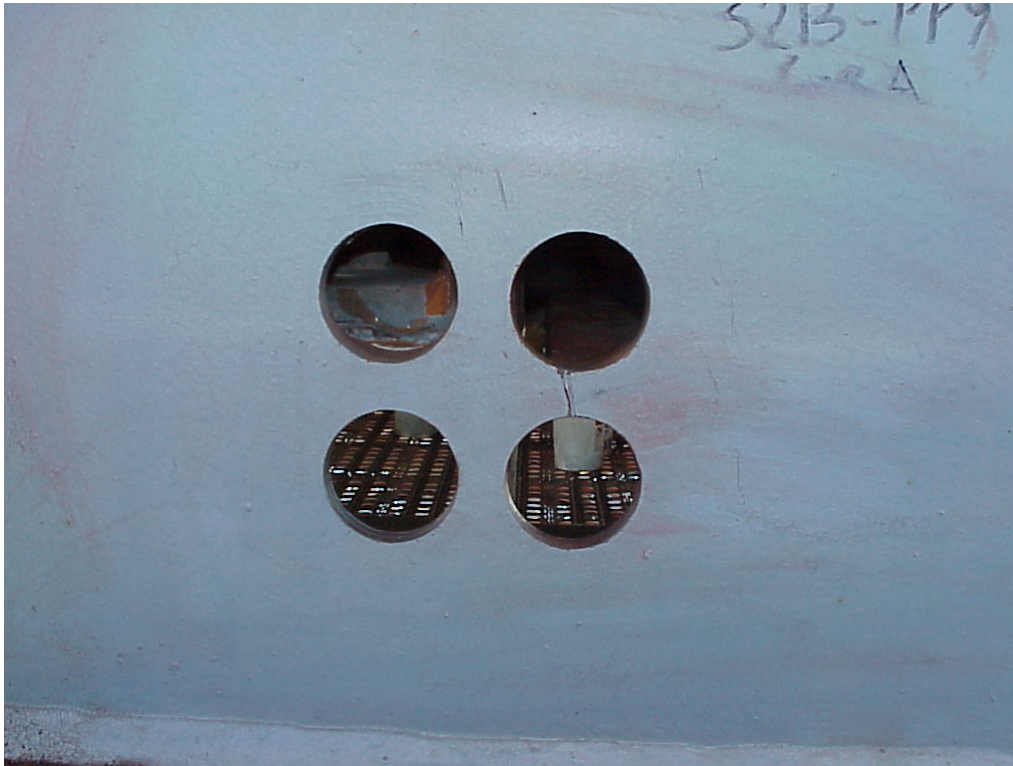
Figure 18 Check holes that arrested CIF crack in gusset weld gap on the I-794 Hoan Bridge.
