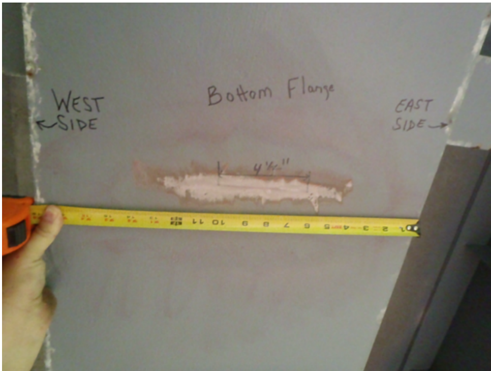
Figure 11 Fatigue crack growth in the lower flange of the girder after the initial web fracture.
