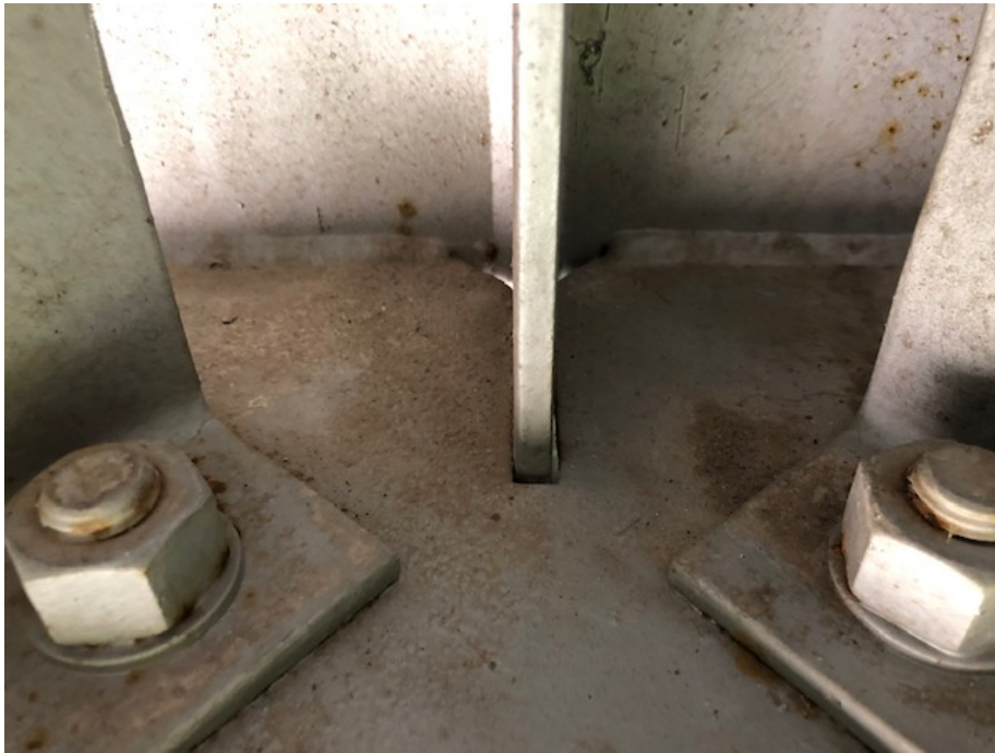
Figure 14 Bridge 045B00049N in Greenup County showing Hoan Detail which is typical throughout entire structure.
