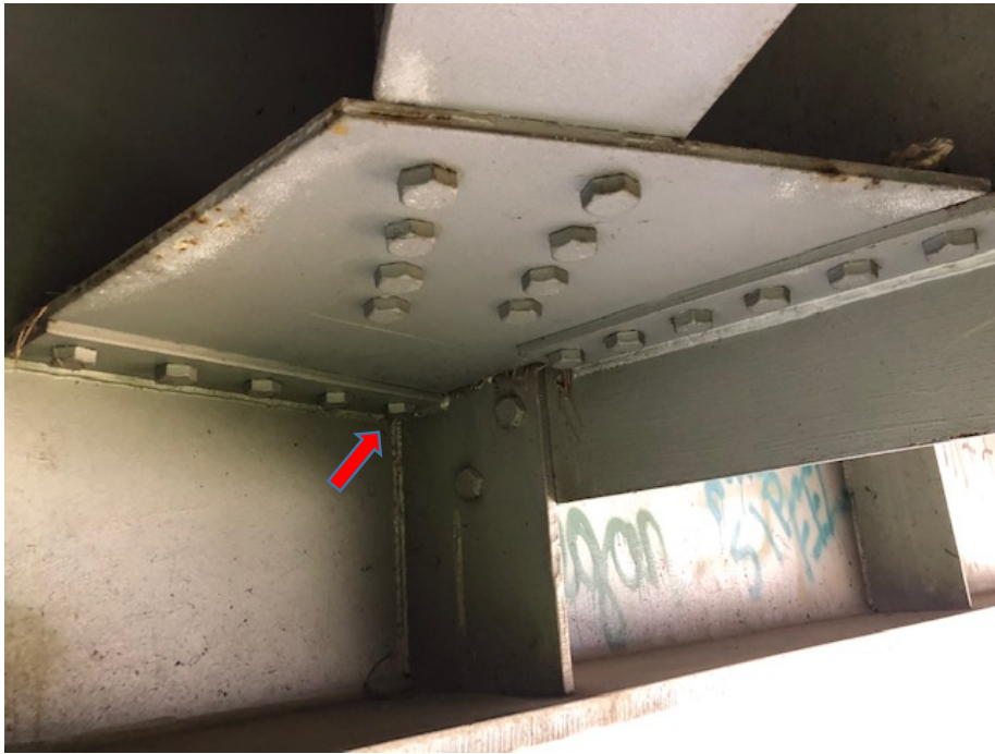
Figure 16 Bridge 040B00028R in Garrard County showing problematic CIF detail related to the gap between perpendicular fillet welds attaching gusset mounting bracket and vertical stiffener to web (arrow).
