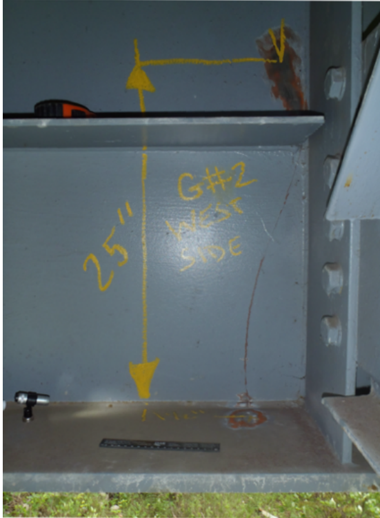
Figure 10 Fracture in interior girder of the northbound I-75 bridge over Lynn Camp Creek in Whitley County (2014).
