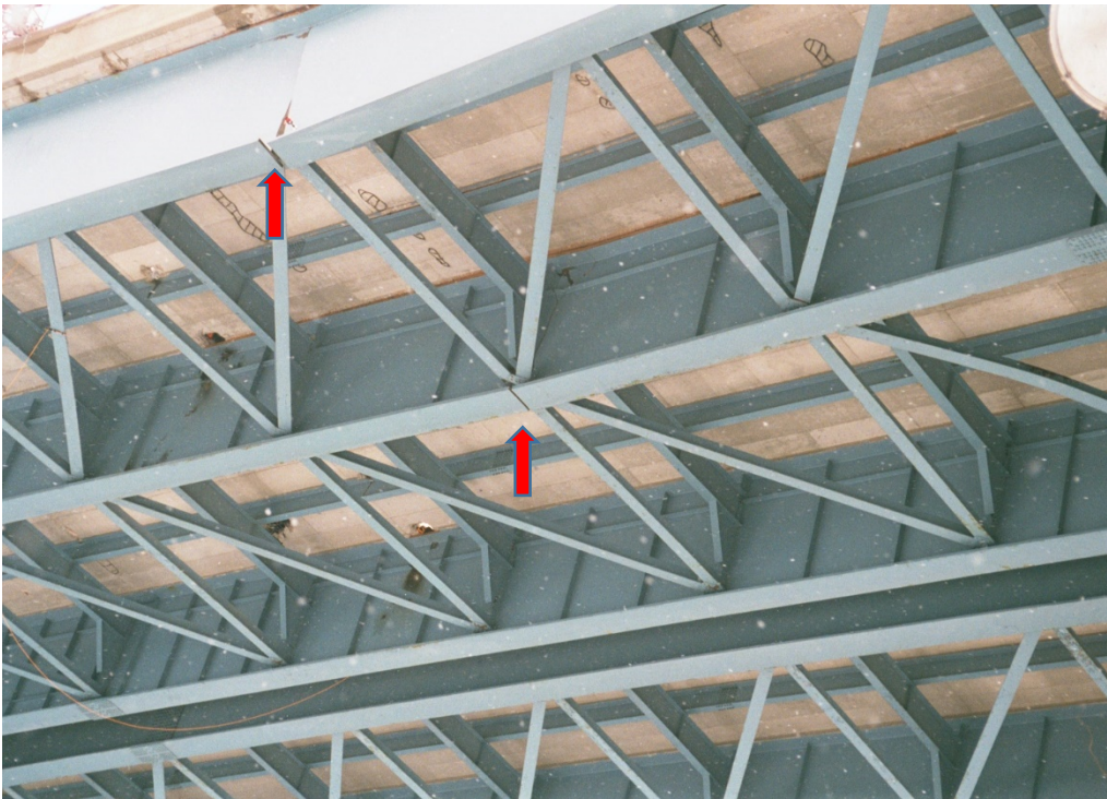
Figure 2 Complete girder fractures in two of the three approach span girders (arrows).
