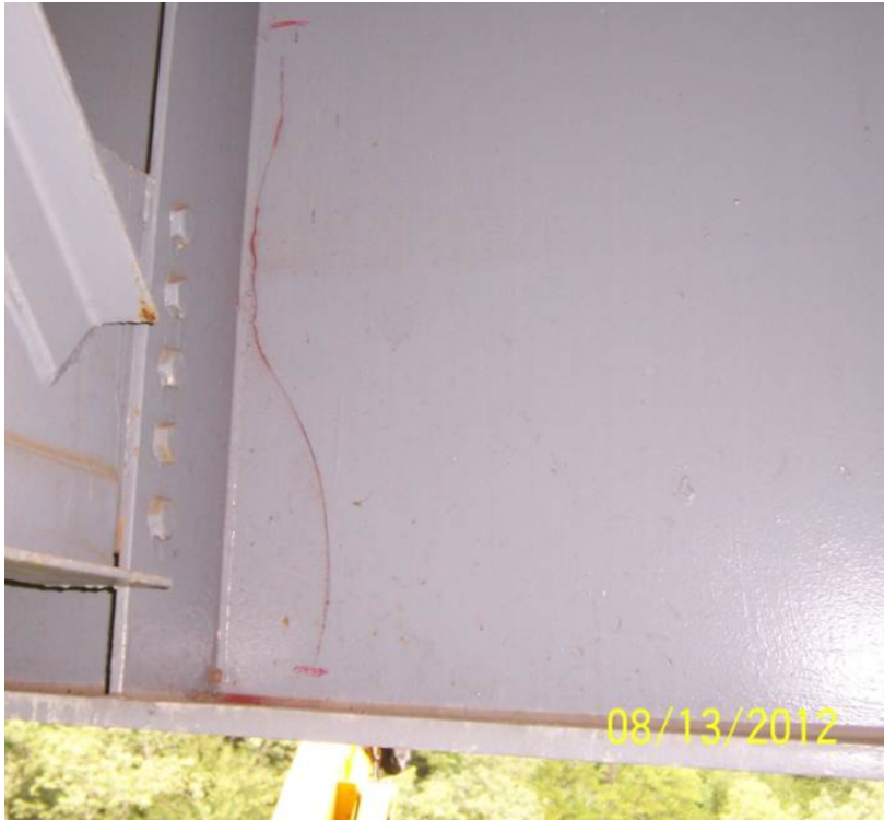
Figure 8 Fracture in interior girder of the northbound I-75 bridge over Lynn Camp Creek in Whitley County (2012).
