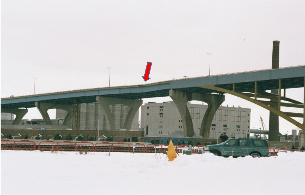
Figure 1 The I-794 Hoan Bridge in Milwaukee, Wisconsin, after the girder fracture event (December 2000). Note the sag in the barrier wall and girder (arrow).
