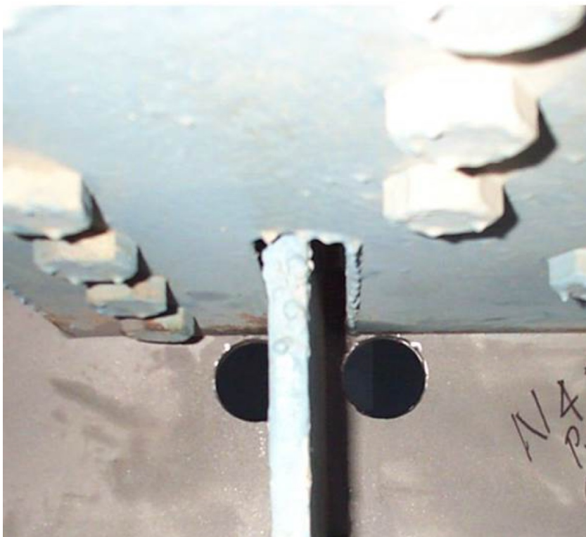
Figure 17 Check holes placed bracketing weld gaps on gusset in the I-794 Hoan Bridge.
