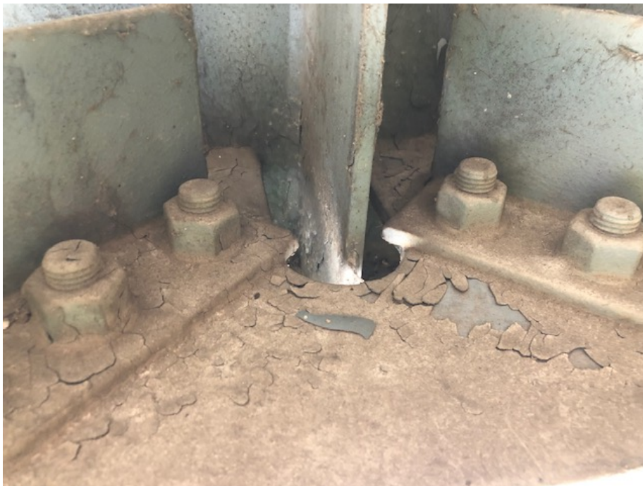
Figure 15 Bridge 073B00120R in McCracken County showing Hoan Detail which is typical throughout entire structure.
