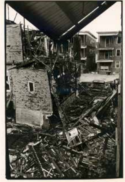
A neighborhood on Hale St, Lowell, MA being demolished as a result of Urban Renewal. Photo courtesy of Tyrrell Richard Schein via archive.org.
