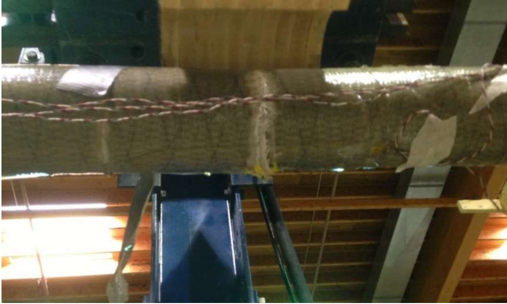
Figure 3-12. Apex Failure Mode
