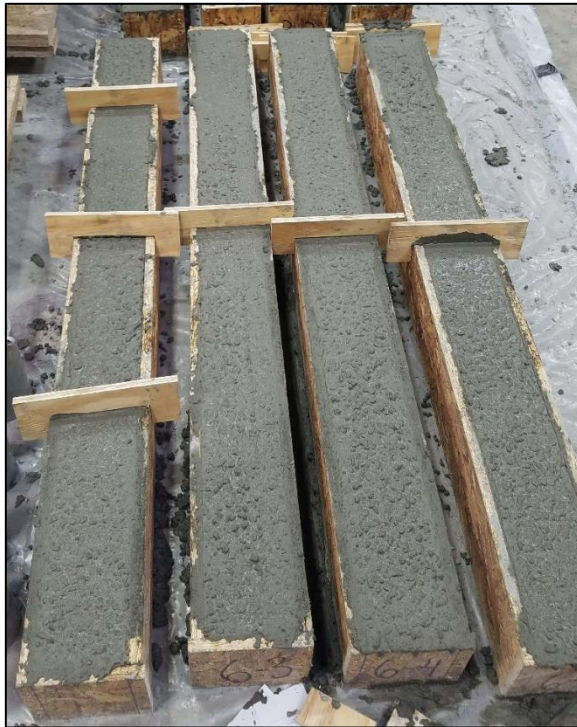
Figure 26: Flat CFRTP panels in formwork before (left) and after (right) concrete pour
