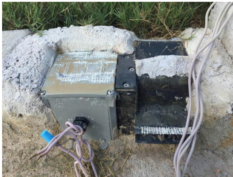
Figure 14. Installed Paddle Wheel Prototype
